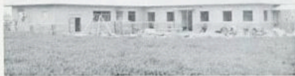
We are just finishing the building for this entirely new Faith, Hope and Love Orphanage. Thirty children have already been gathered from the streets of Taegu and are being cared for temporarily in another building. The orphanage will be formally opened this month (June). Mr. Lee Sang Young, a new Christian, gave a fine piece of the best rice land in the area and some cash. In this way he is showing his gratitude to God for salvation! ESEA provided $6,000 and will sponsor all the children.
